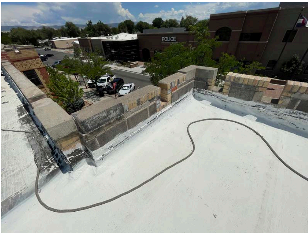
Photo 37: Parapet, south side of building at original building parapet (left side) meeting western section of building parapet and where bricks were reused. Newer parapet has larger cinder or CMU type blocks.
