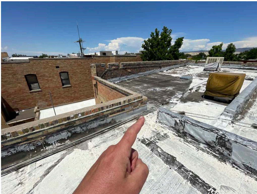
Photo 39: Low point for primary roof to drain. Water then moves north to scupper/drain.
