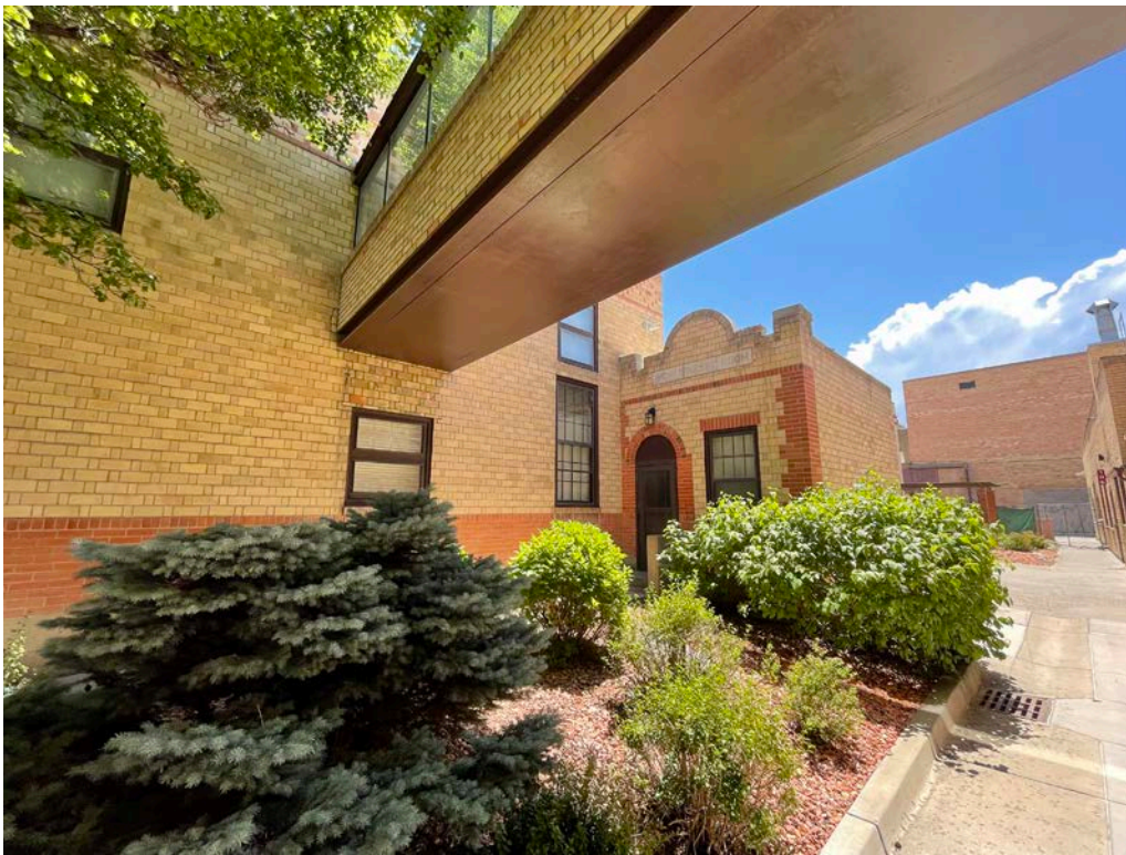
Photo 44: View southwest, sky bridge above, north exterior elevation, historic entry point to restrooms.
