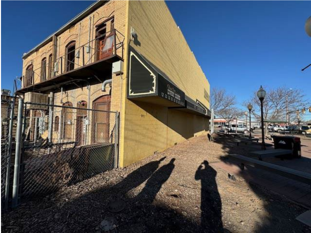
East side. These lots (now Demoret Park) used to have another building abutting the Sherman and Ross Block Building, which burned down. As a result, this side was not historically exposed, and this is not original.
