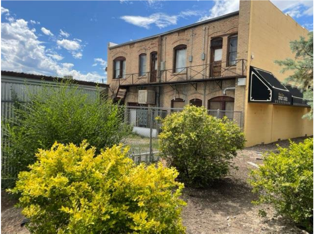
Rear side. Note that there has been a recent addition attached to the rear. Windows and doors have segmental brick arches and stone sills.
