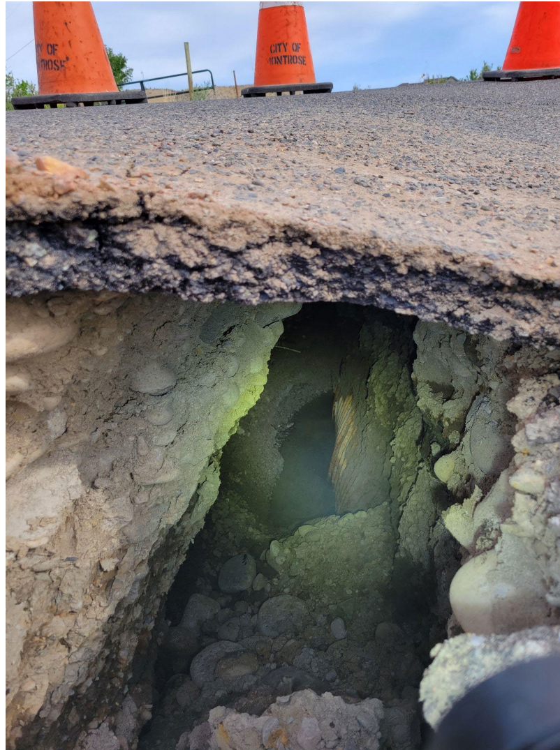
Photo 3: Looking in the hole under the Roadway. Observe the length and depth of the undermining.
