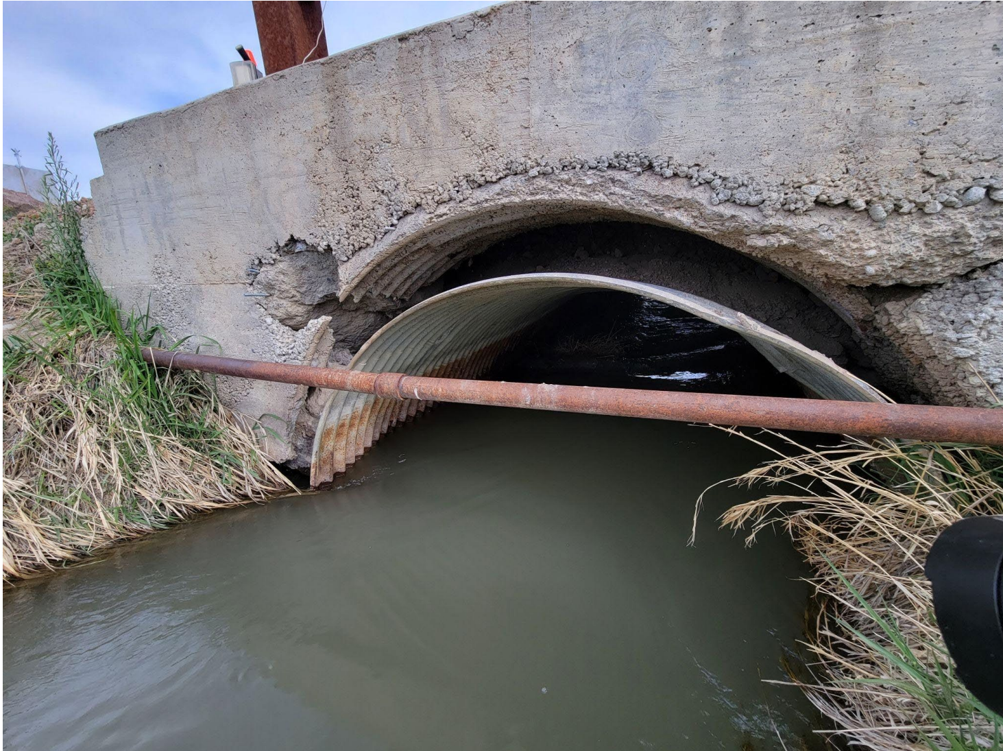
Photo 4: 1'- 1' 6" of separation from headwall due to collapse of culvert.
