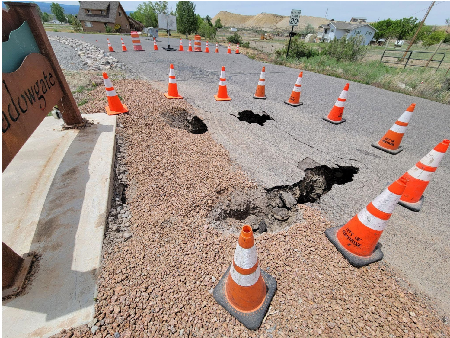
Photo 1: Roadway's Condition After First Call of Reported Damage
